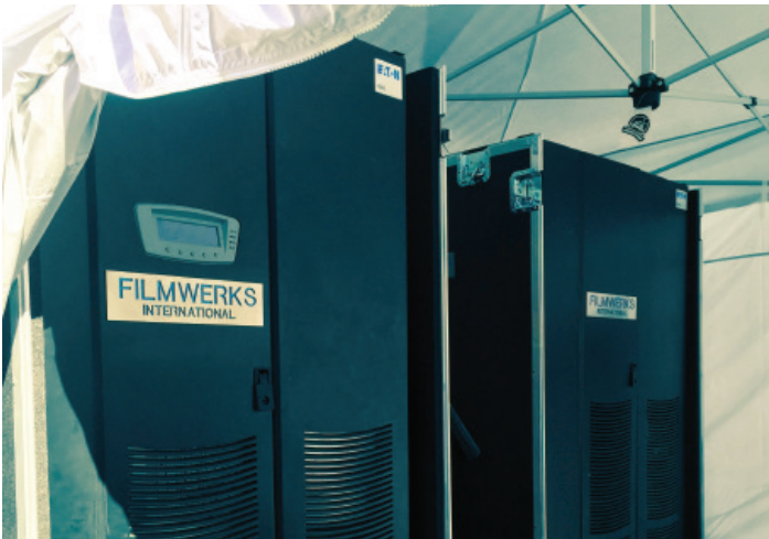
Filmwerks technicians begin preparation for the Super Bowl by setting up an Eaton UPS.
