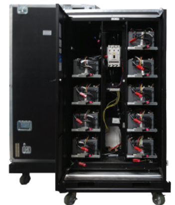
It's critical that all the technology is portable and road-friendly. Here UPS batteries are on casters to easily transport into the stadium.
