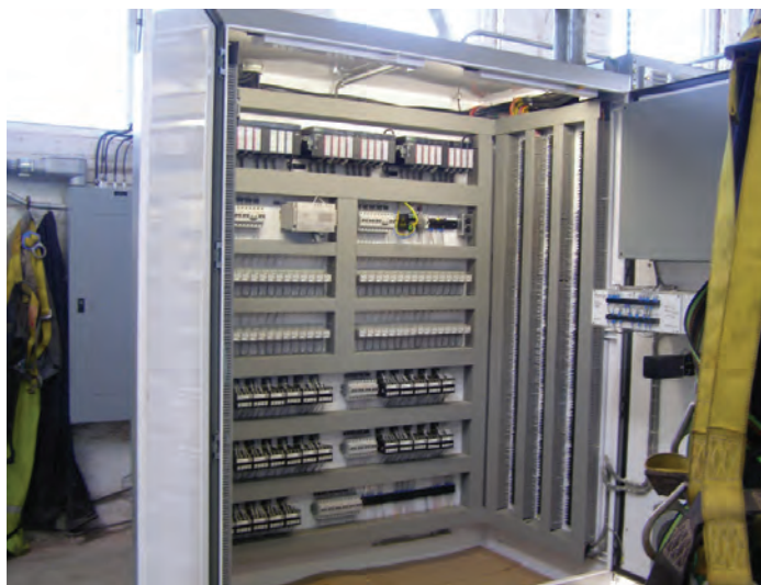
PLC panel for small hydro
