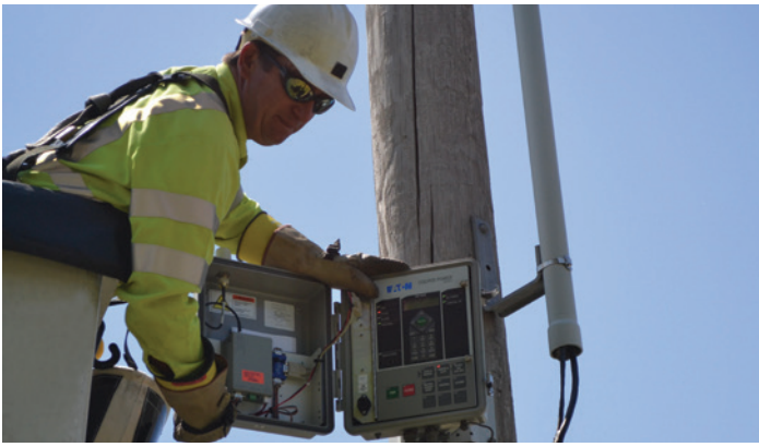
KCP&L lineman installing and field testing automated capacitor control on distribution capacitor bank
