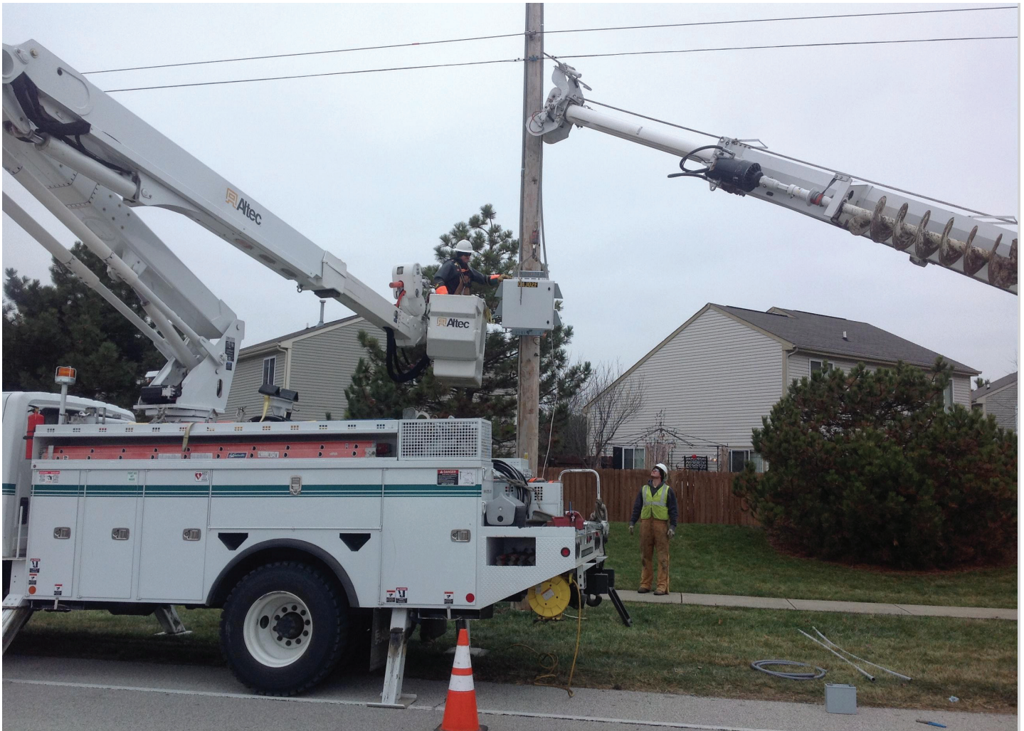
With its new AMI system, Johnson County REMC can perform outage detection in near real time to expedite repairs
