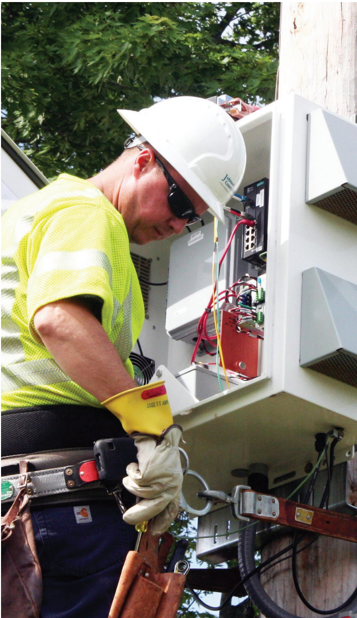
A Johnson County REMC communications technician installs the utility's new two-way advanced metering infrastructure
