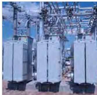
Substation voltage regulators with controls
