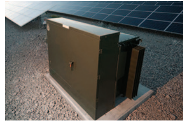
Medium voltage step-up transformer
