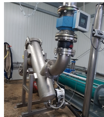
In the sewage treatment plant, the fully automatic MCS-500 strainer basket filter replaces a manual solution that cost the operating staff several hours of work every day.
