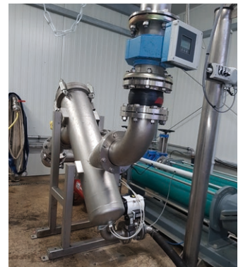
In the sewage treatment plant, the fully automatic MCS-500 strainer basket filter replaces a manual solution that cost the operating staff several hours of work every day.
