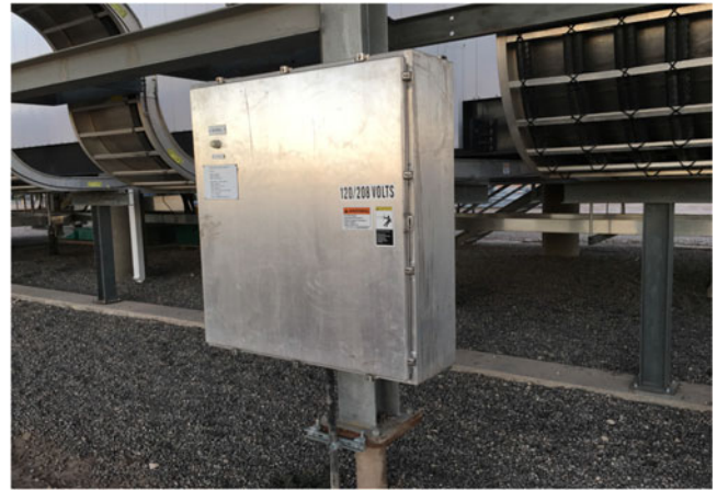
Fig. 10. CPT switched resistor control cabinet.
