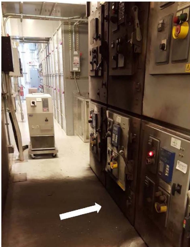
Fig. 1 Motor control center after fault
