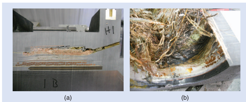
FIGURE 3. A cross section of the line-end VT failure: (a) the VT high-voltage side and (b) the VT windings.
