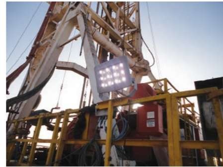
HAZARDOUS AREA LED FLOODLIGHT INSTALLED ON A RIG
