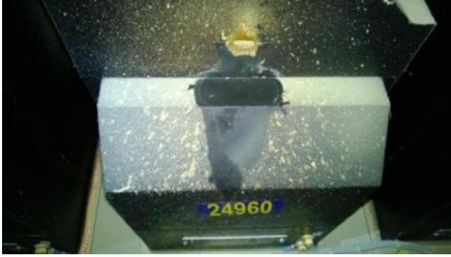
Fig. 2. Line-End VT Failure
