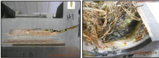
Fig. 3. Cross Section of the Line-End VT Failure
