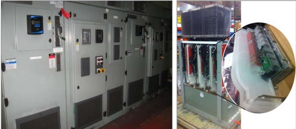
Fig. 6: Two of the new AFDs installed at left, inverter sub-assembly showing silicone-encapsulated power pole at right.
