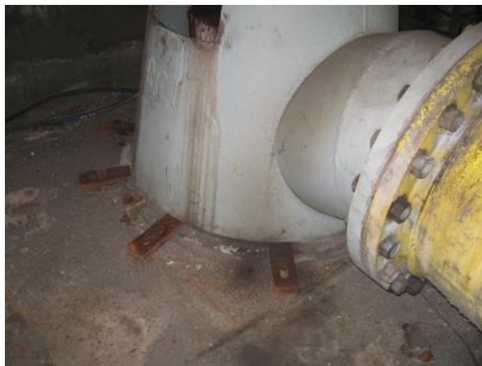
Fig. 7: New pump mounting clamps added to the existing vertical ROT pumps.
