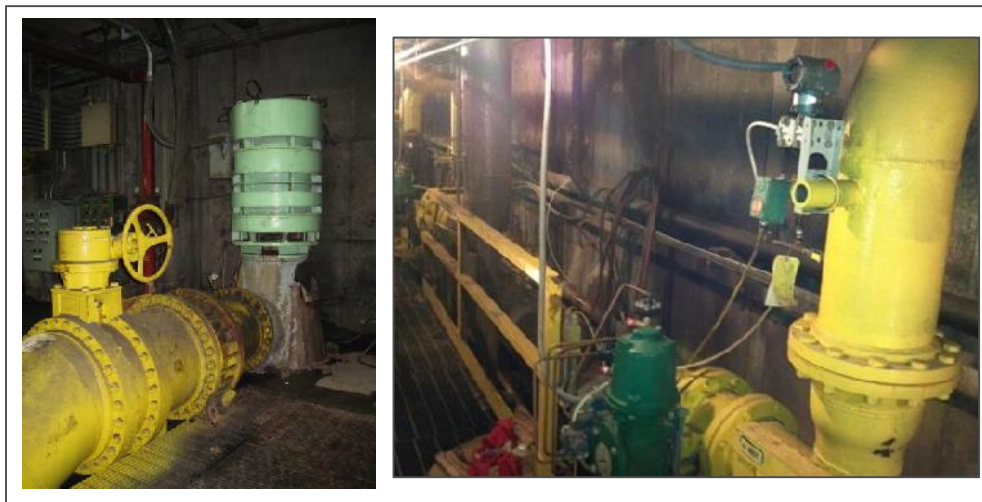
Fig. 2: One of five 15,000-GPM ROT pumps at left, control valve and installed bottom bank pressure transmitter at right.
