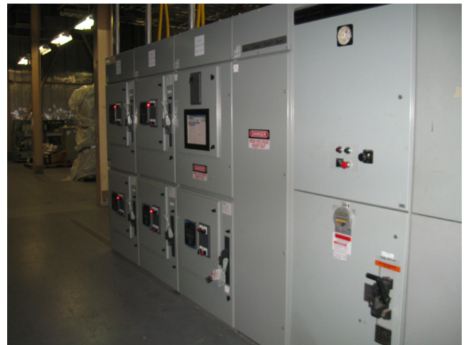
Fig. 7: The 1970's vintage MCC structures at the right, followed by a bus transition section and three new MCC structures at the far left.
