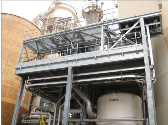
Fig. 1: New Bleach Plant Wash Press stage 1. Rotary drums and motors installed on upper steel platform.
