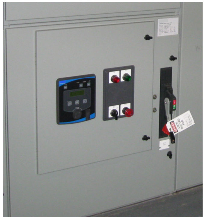
Fig. 10: Each starter cubicle includes a starter display module (SDM). Door mounted discrete control devices were included for ease of interface to the existing DCS
