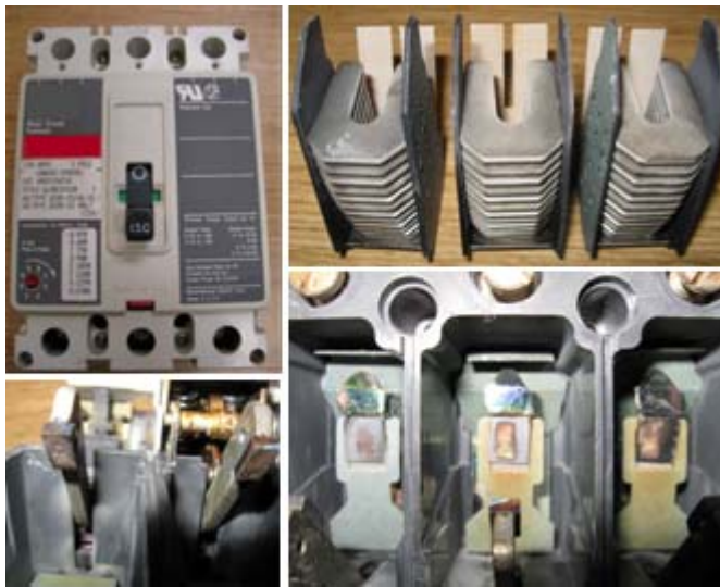
Fig. 10: Photos of Breaker 4919-4 clockwise from upper right; external breaker case, arc-chute assemblies, main moving and stationary contacts with evidence of elevated heat primarily on Phases B and C, close-up of Phase C moving contact.
