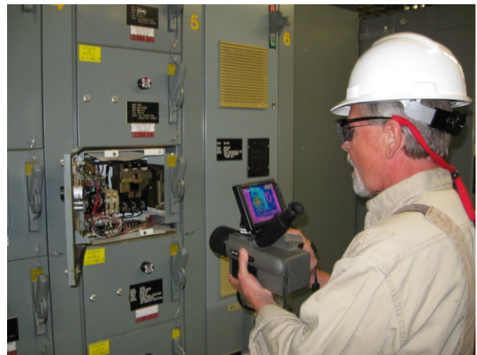
Fig. 6: Paper mill Thermographer conducting thermal scan survey of low-voltage MCC compartment.
