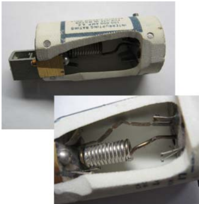
Fig. 15: Photo of current-limiter removed from service from Paper Machine #1 area. Cutaway view shows three elements melted while one remains intact.
