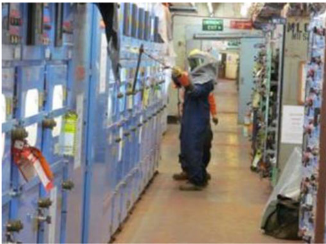
Fig. 2. Performance of circuit breaker operation during isolation for this vintage switchgear presents a significant risk to personnel.
