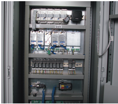
Figure 1. Cubicle MR90 system (fixed station).
