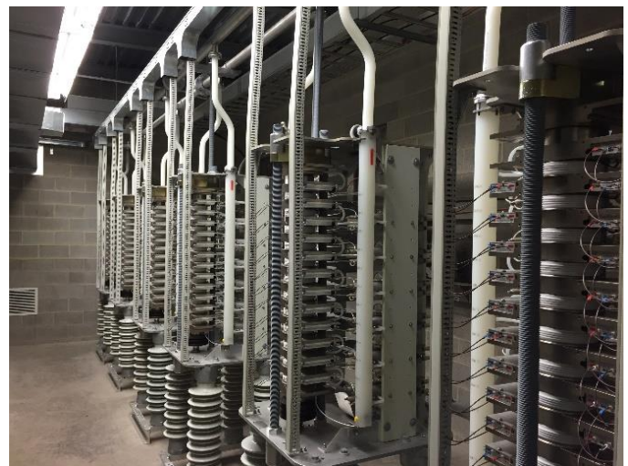
Figure 7. TCR Switch View – Two (2) Stacks of Twelve (12) Thyristors per Assembly for a Total of Twenty-four (24) per Phase
