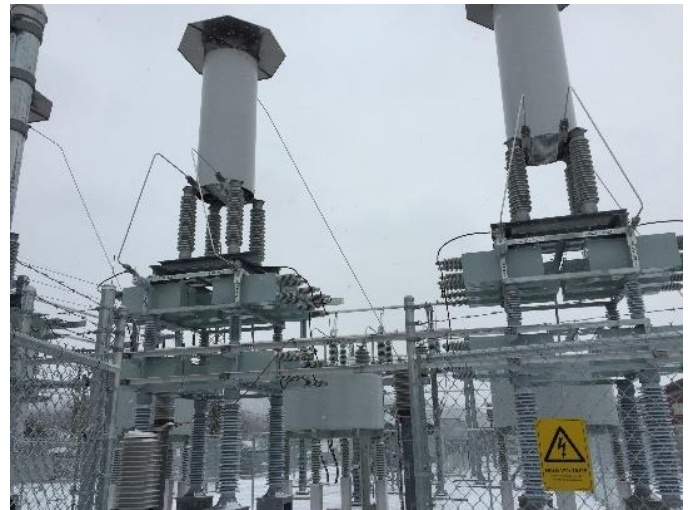
Figure 6. Standard Steel 2nd Harmonic Filter – C- Type Filter viewing Capacitors, Tuning Reactor and Damping Resistor
