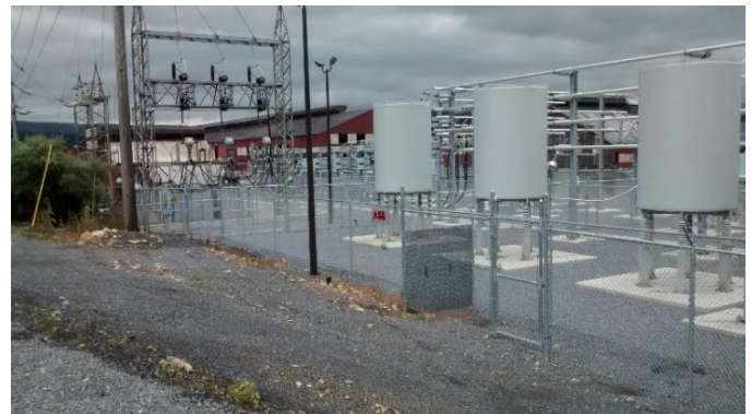
Figure 13. Completed SVC Substation – View encompasses Incoming 46 kV from plant, TCR Reactors and filter banks in background
