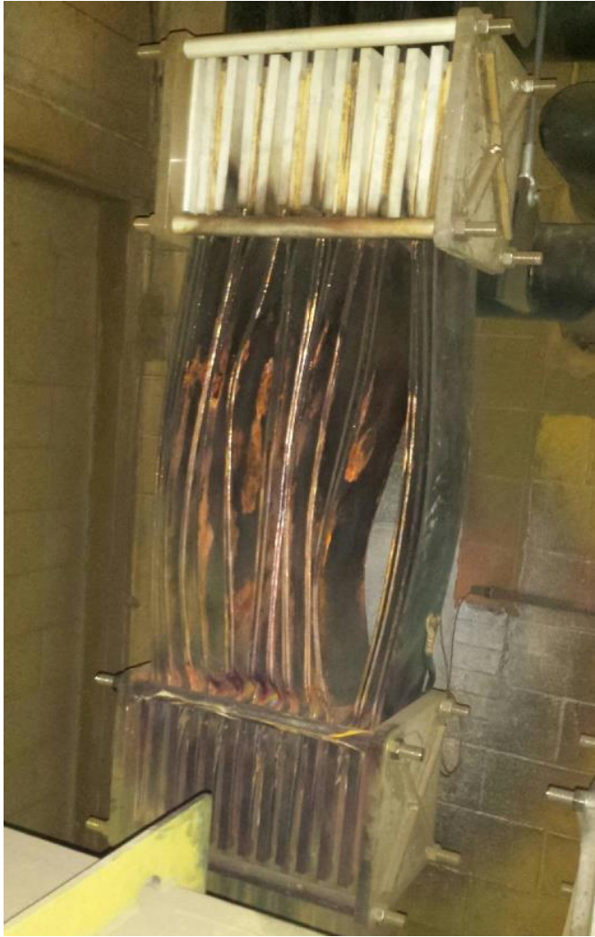
Figure 14. EAF#4 Delta Closure damage shortly after SVC went online
