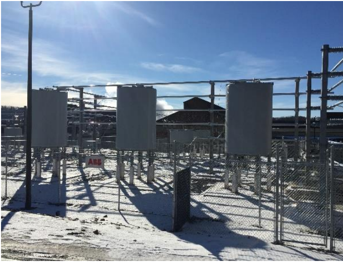
Figure 8. TCR Reactor view – Presenting three (3) Main Reactors, one per phase, located outside the TCR Switch Room
