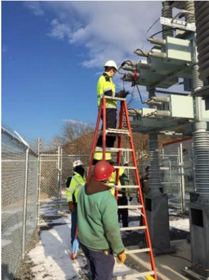
Figure 11. SVC 2 nd Harmonic Commissioning – Verifying Capacitors
