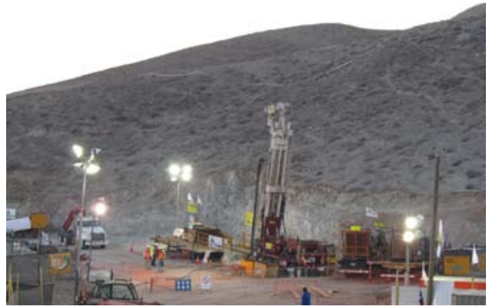
The towering Schramm T130XD drill rig took center stage outside the mine.
