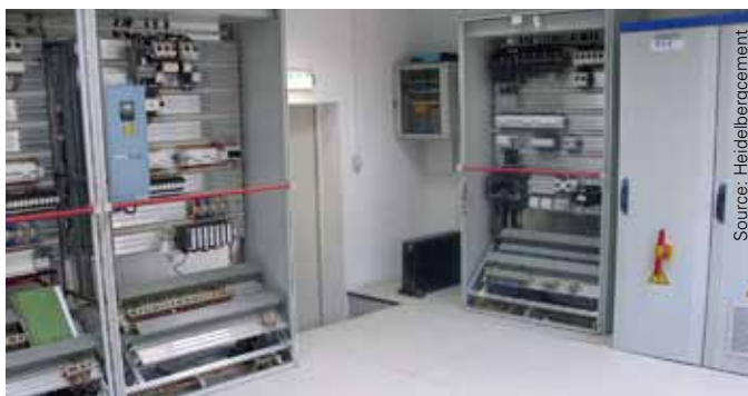
To control the new motors, Eaton SPA/SPI 9000 series VSD were selected for the inclined conveyors, and Eaton SPX series VSD for the horizontal conveyors; these were built into control panels based on floor-standing cubicles from the Eaton xVTL range
