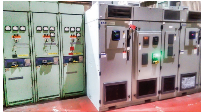
New Eaton drives (right) next to existing starters.
