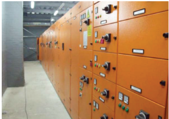
First floor MCC completed and fully functional
