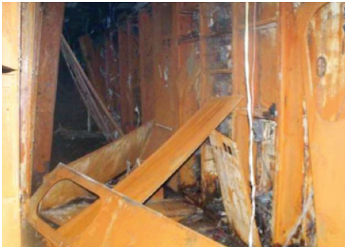
First floor Motor Control Centres - irreparable
