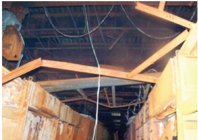
An unrecoverable MCC
