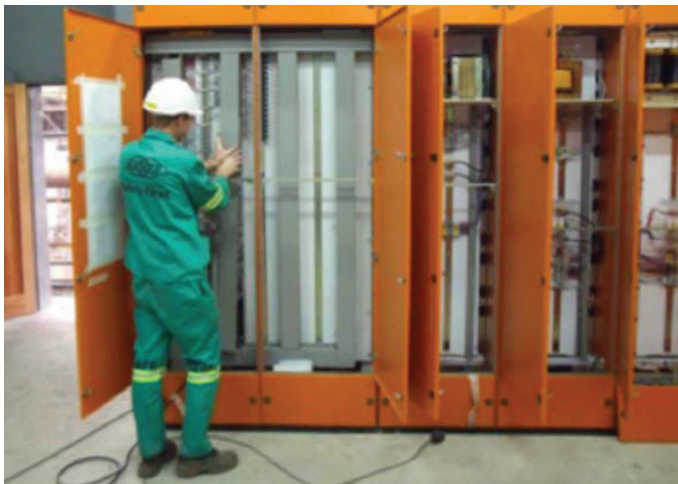
Stage one of the new Motor Control Centres being commissioned
