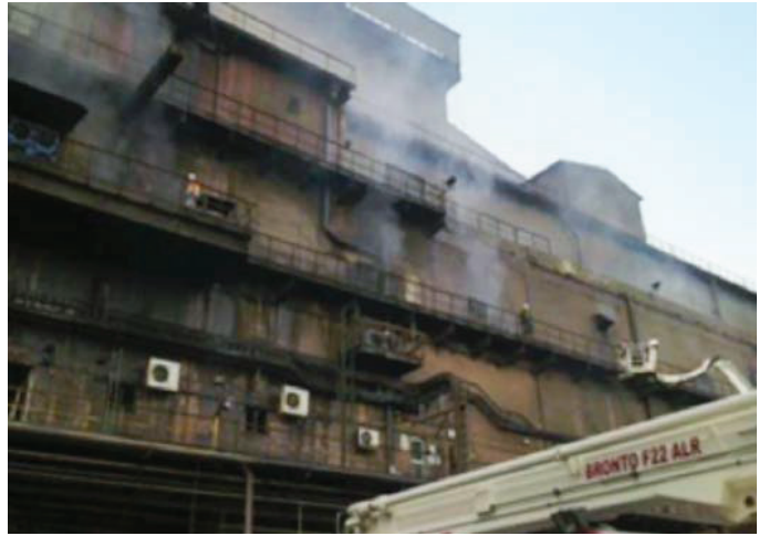
First and second floor control rooms burnt to ruins
