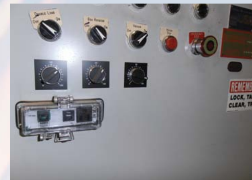
Figure 2: This remote port can be used for equipment programming. This permits the equipment to be programmed by the worker without wearing electrical PPE and without specialized electrical safety training. Courtesy: MES Consulting Services
