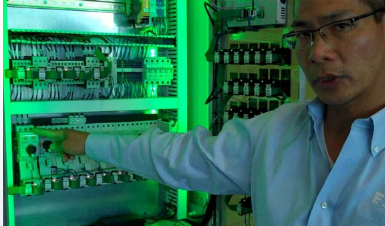
Machinery original equipment manufacturers and their customers can take advantage of remote diagnostics with web server capability on the controller and easy connection via Ethernet to the Internet to limit downtime. Courtesy: CFE Media
