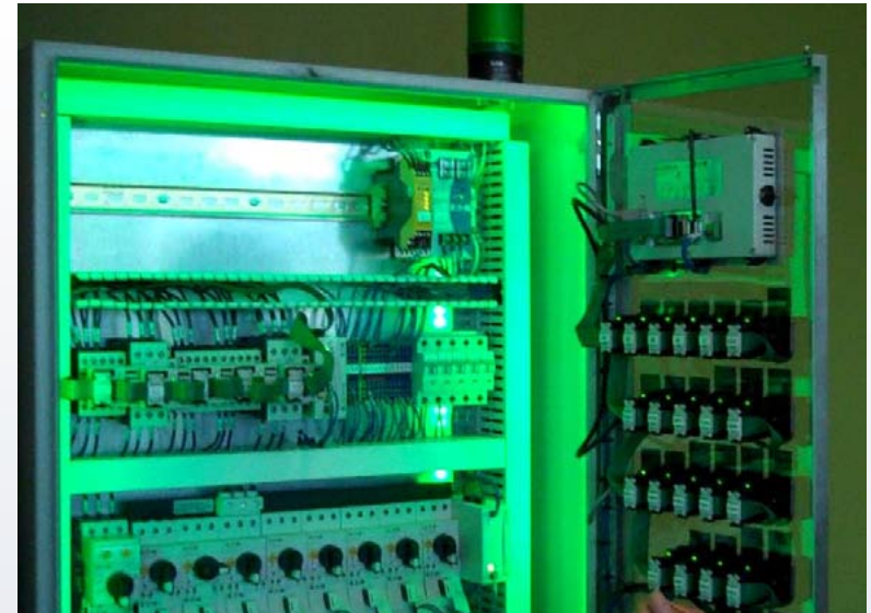
A trip condition can provide a local alarm indication and notification via the Internet. In an overload situation, the contactor can open, disconnecting the load before the circuit breaker can trip, so a remote restart is possible without a visit to the enclosure. Courtesy: CFE Media
