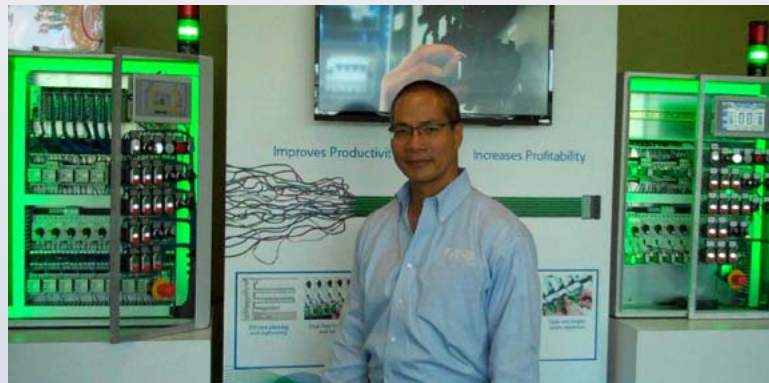
Lean automation helps streamline control panel design on the right, producing overall savings of 35% and build time savings of 60% or more. Richard Chung, product manager, lean automation, Eaton, explains to CFE Media's Mark T. Hoske how the Eaton SmartWire-DT system helps with that, at the Eaton Menomonee Falls, Wis., facility. Video is about 9 minutes. http://www.controleng.com/single-article/control-panel-before-and-after-gain-productivity-with-lean-automation-connectivity/b457ded5a1611d12644a2532865082d4.html Courtesy: CFE Media
