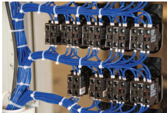
Figure 2. Additional control panel construction time is required when wiring is bundled to door-mounted devices because wires must not restrict opening and closing the door.
