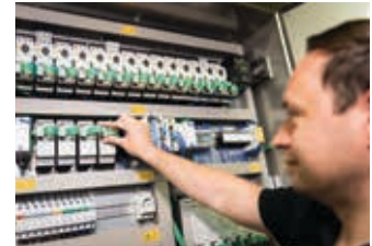
Thanks to the SmartWire-DT intelligent connection and communication system the wiring is reduced by approximately 40%
