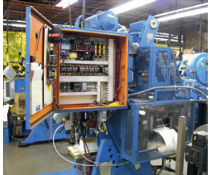
This machine's industrial control panel has 50 kA SCCR marked on the nameplate inside the enclosure. The available short-circuit current is field marked on the exterior.
