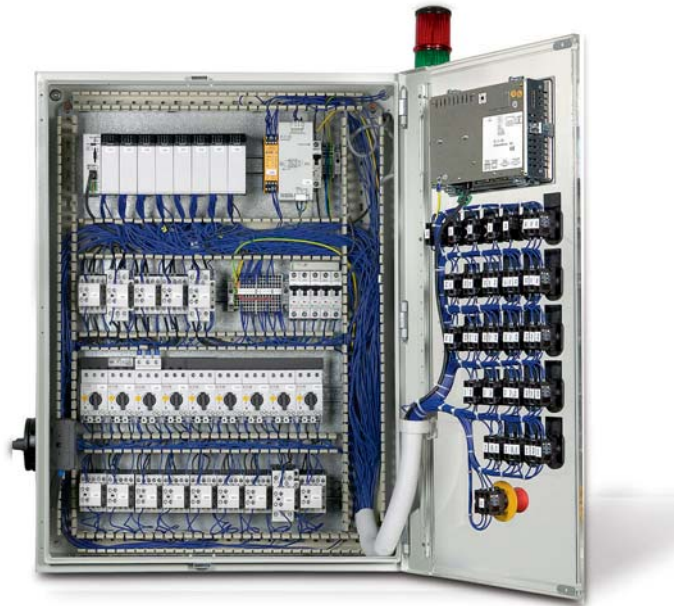
Figure 4. Control Cabinet Before
