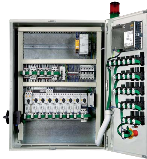
Figure 5. Control Cabinet After a Device-Level Network like Eaton's SmartWire-DT® System Connects Devices, While Eliminating the Hassles of Traditional I/O Wiring.
