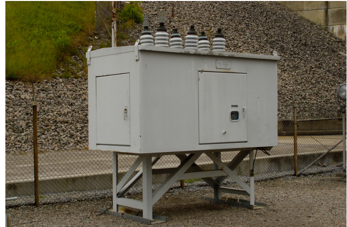
Figure 7. Spare Conversion Circuit Breaker
