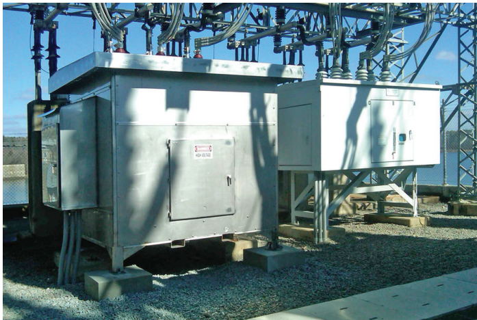
Figure 8. Second Conversion Circuit Breaker and First Conversion Circuit Breaker
