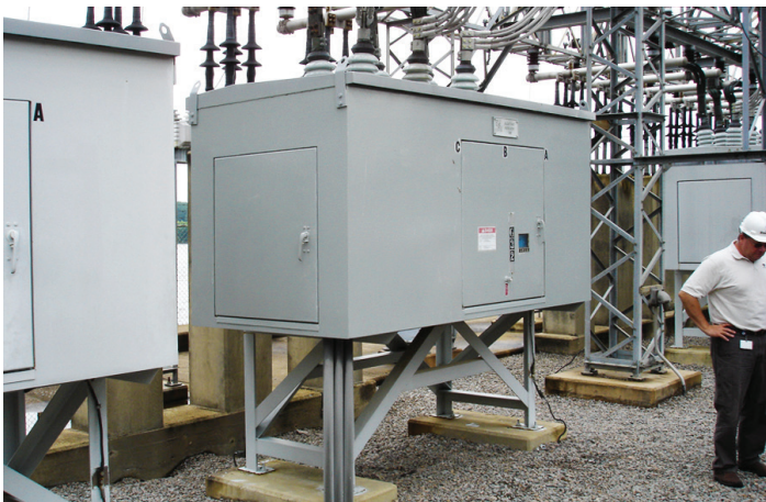
Figure 6. First Gaston Circuit Breaker Conversion
