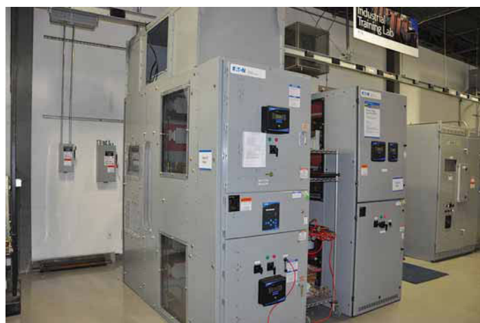
Medium voltage switchgear
