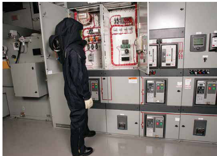
Worker wearing PPE inspecting low voltage switchgear
