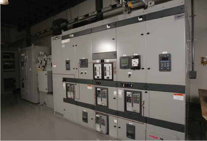
Low voltage switchgear
