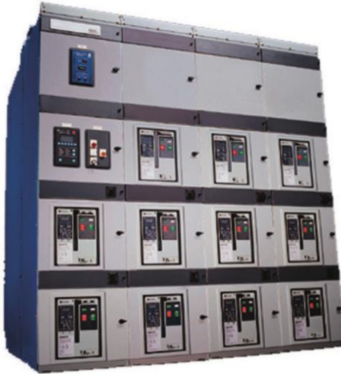
Figure 3: An Arcflash Reduction Maintenance System shortens fault clearing times by bypassing time delays in the trip circuit.
