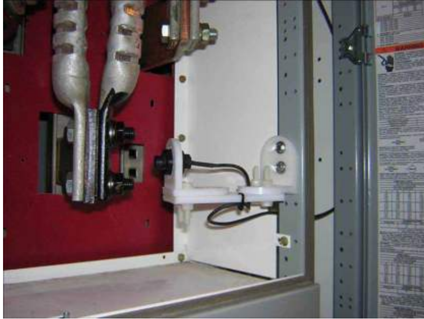
Figure 4: Pyrometers, like the one shown here, continuously monitor pressure junctions for signs of loosening.
