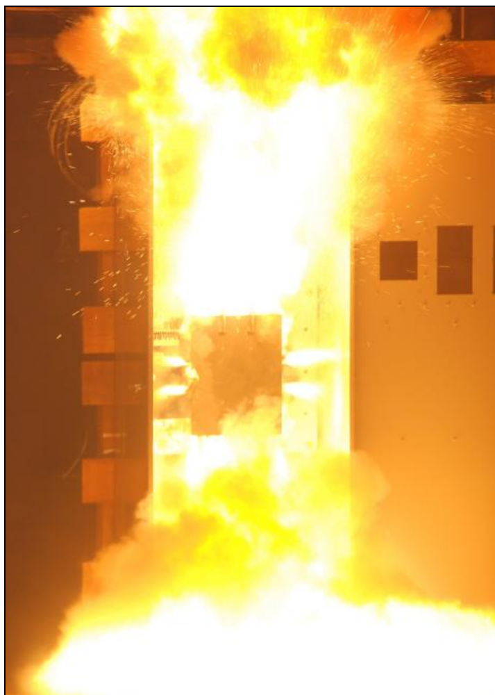
Figure 1: In a data center, arc flashes can ignite large and dangerous explosions.
