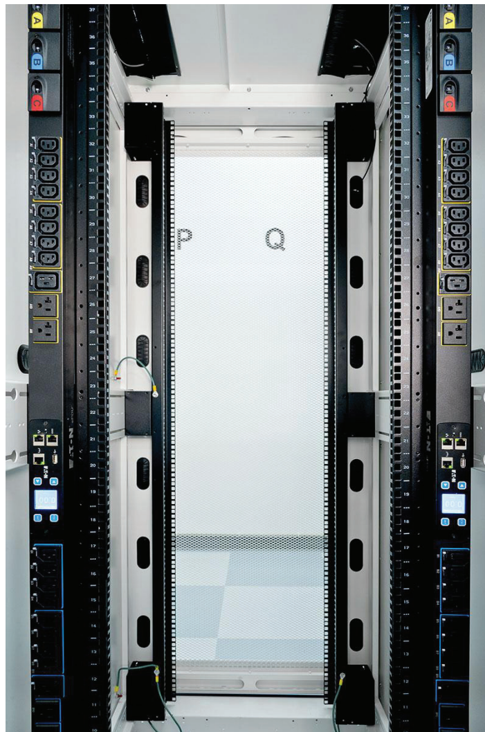
VTC selected Eaton's easily manageable and highly reliable G3 ePDUs to facilitate their model of metering and billing power at actual use with utility grid accuracy.
