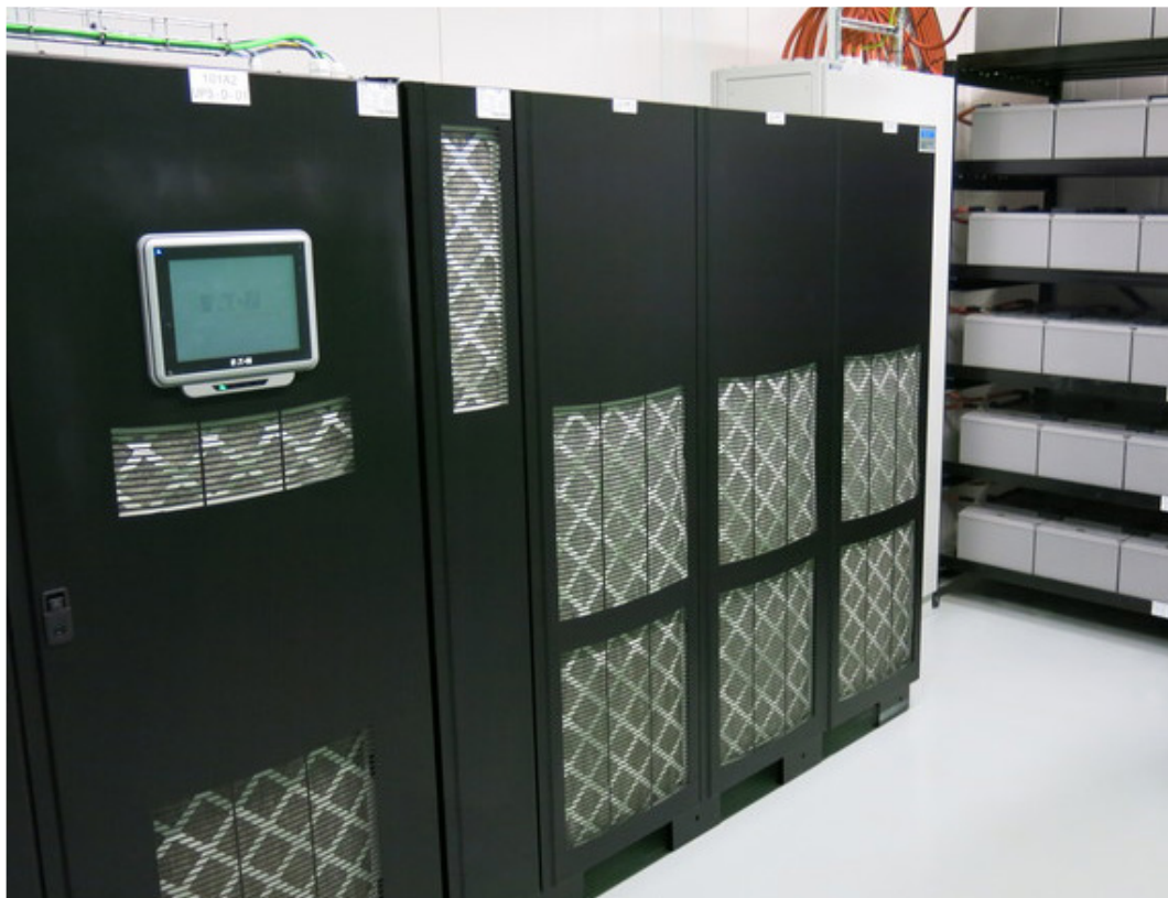
Power Xpert 9395P and batteries
