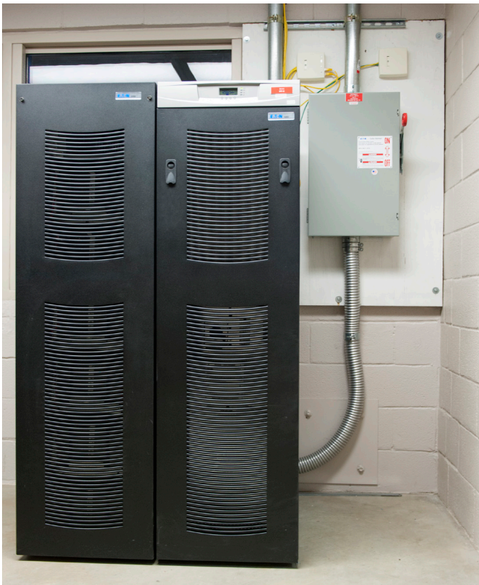
Eaton 9355 and External Battery Cabinet with 9355 General Duty Safety Switch
