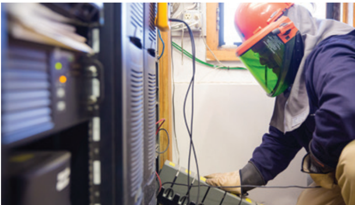
We safely removed 32 trays of batteries and two cabinets—about 3,840 pounds of materials.
