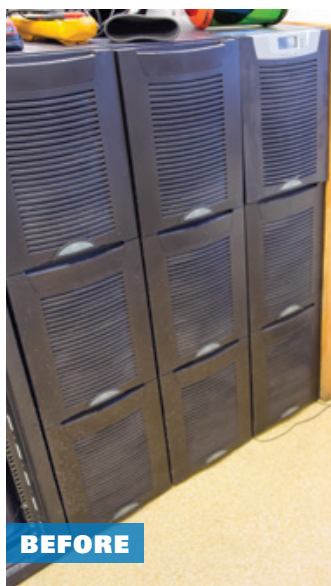
We helped MWO significantly consolidate its UPS, saving valuable space at the summit.
