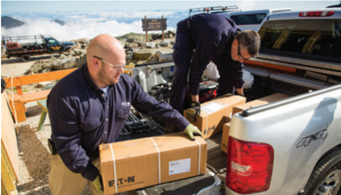
The replacement involved installing four new strings of batteries and removing the other two cabinets and their batteries.
