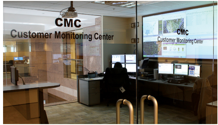
Customer monitoring center
