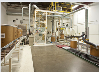
Chemical manufacturing plant
