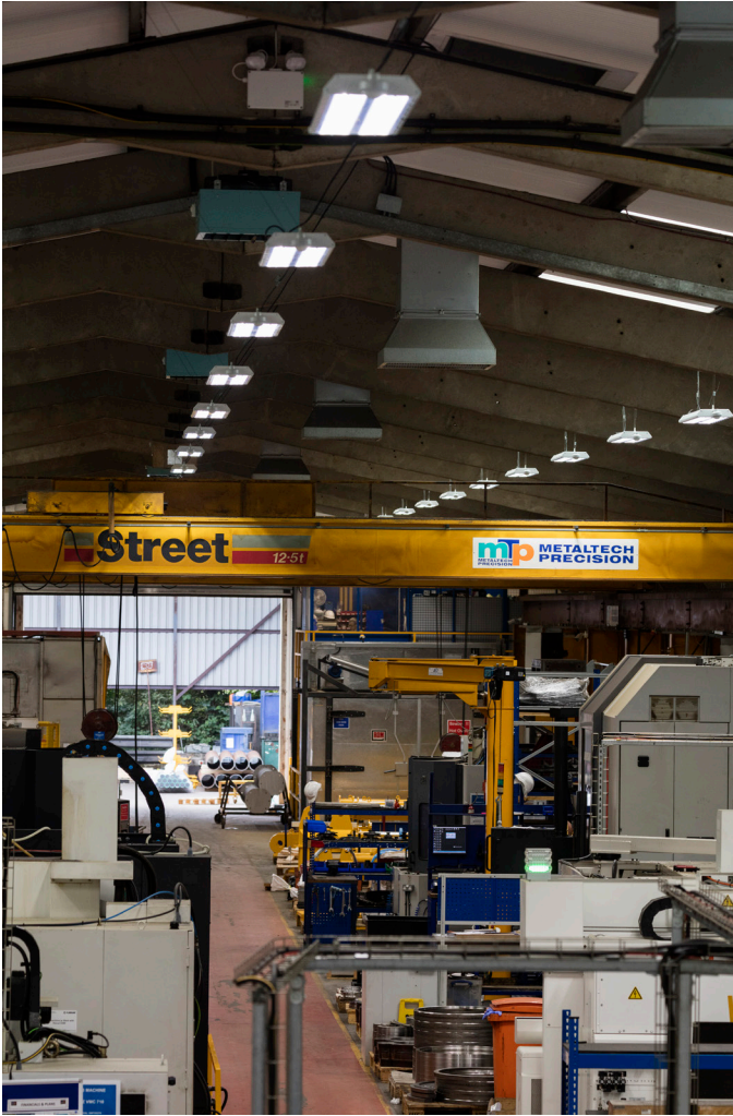
Metaltech Precision sub-contracting plant application of Litex Elite
