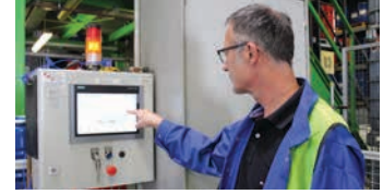
With the use of various operator panels spread across the system, to which the SmartWire-DT system communicates the information, the employees can see when and why a fault or downtime occurs
