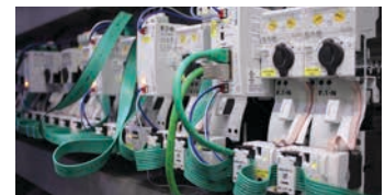
Via gateways, SmartWire-DT can be connected with all standard fieldbus systems, e.g. with Profinet as at BASF
