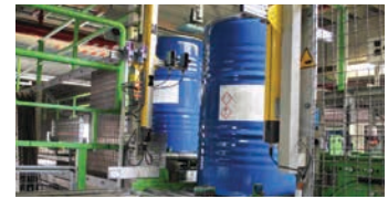
Within the framework of the project, the automation technology of the barrel transportation system at BASF was upgraded with its 50 drives
