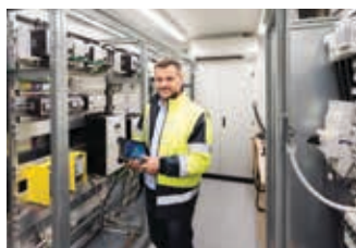
Weingärtner's Philip Fels: "Every drive in Iffezheim is now monitored by SmartWire-DT, so we have valuable capacity utilization information on the thermal motor image."
