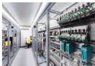
The control station and the electronic technology were shipped in one container so that the crushing operation modernization project could be completed as quickly and smoothly as possible.
