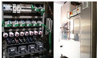
The green SmartWire-DT wiring in the switch cabinet not only saves space and time, but also allows for the detailed documentation of all operations.
