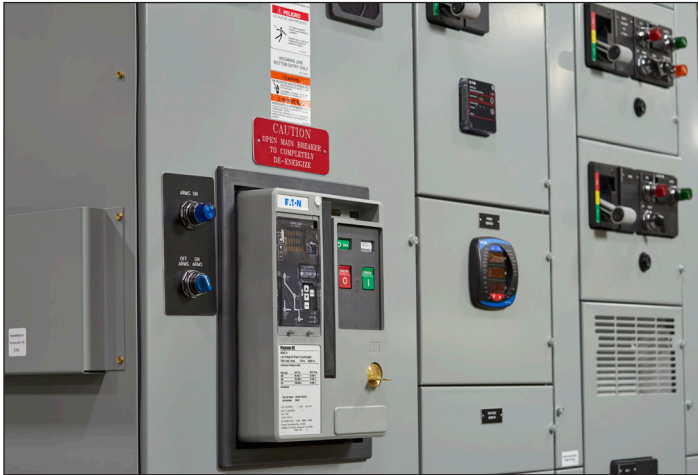
Figure 2. A typical low-voltage motor control center shown above.
